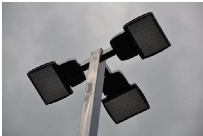
Regency Centers installed LED lights at the parking lot of the firm’s Willston Centre II.
